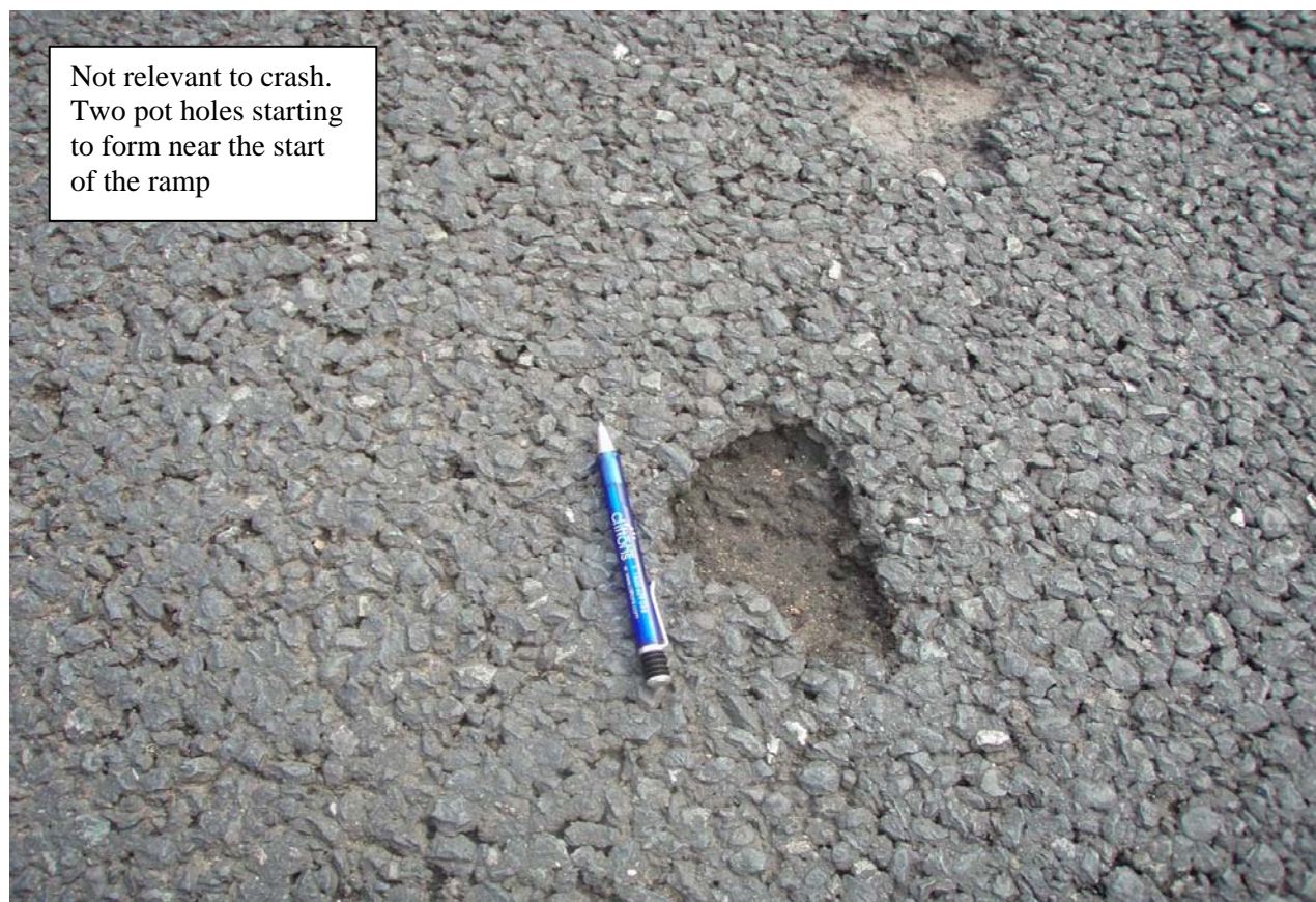
Photo 14 – Small pothole starting to form near start of ramp
