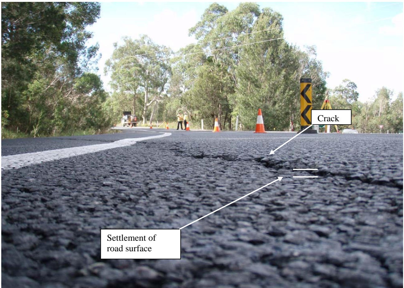
Photo 11 – Settlement of road and environmental crack in pavement
