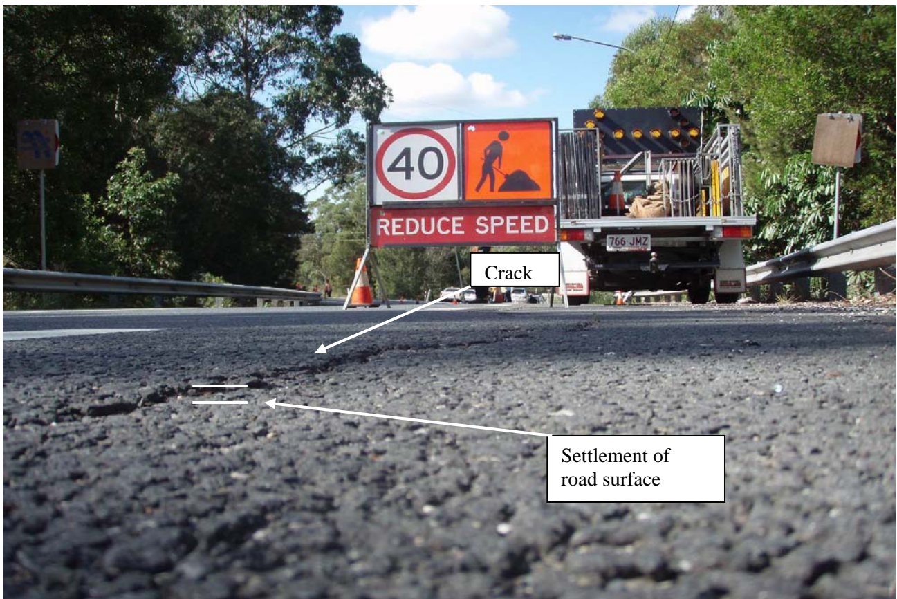
Photo 12 – Settlement of road and environmental crack in pavement
